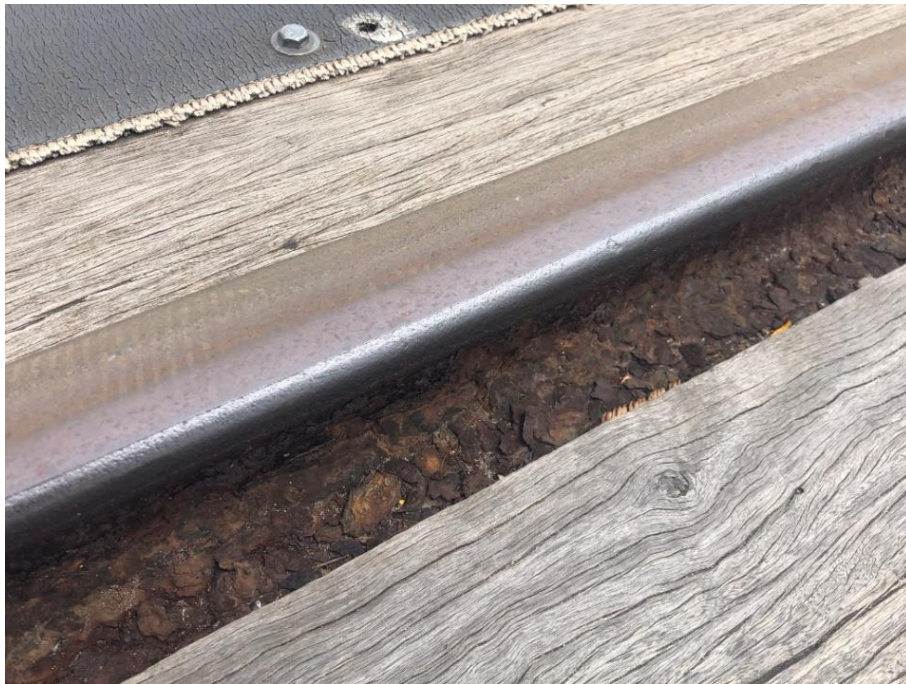
Figure 3.2: Corroded Rail Foot and Web
