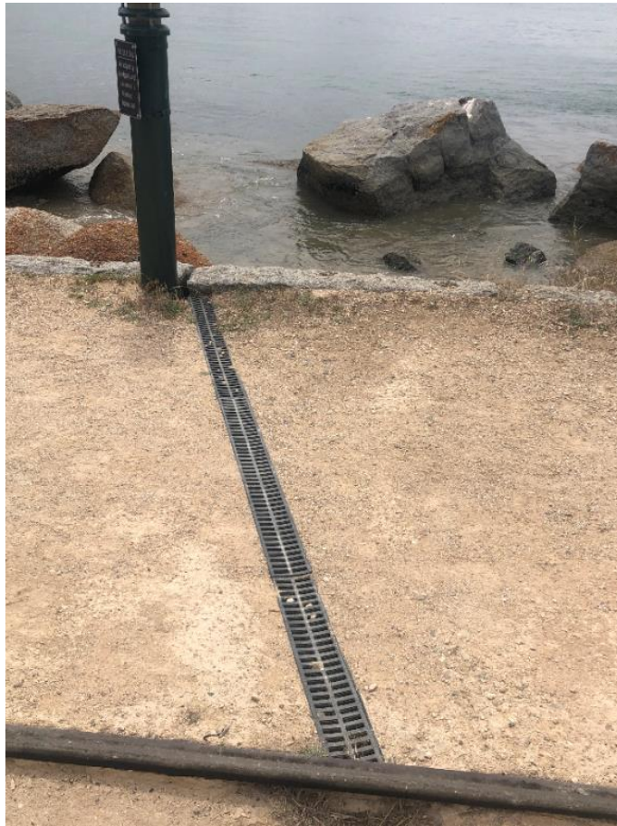
Figure 3.5: Typical Grated Drain
